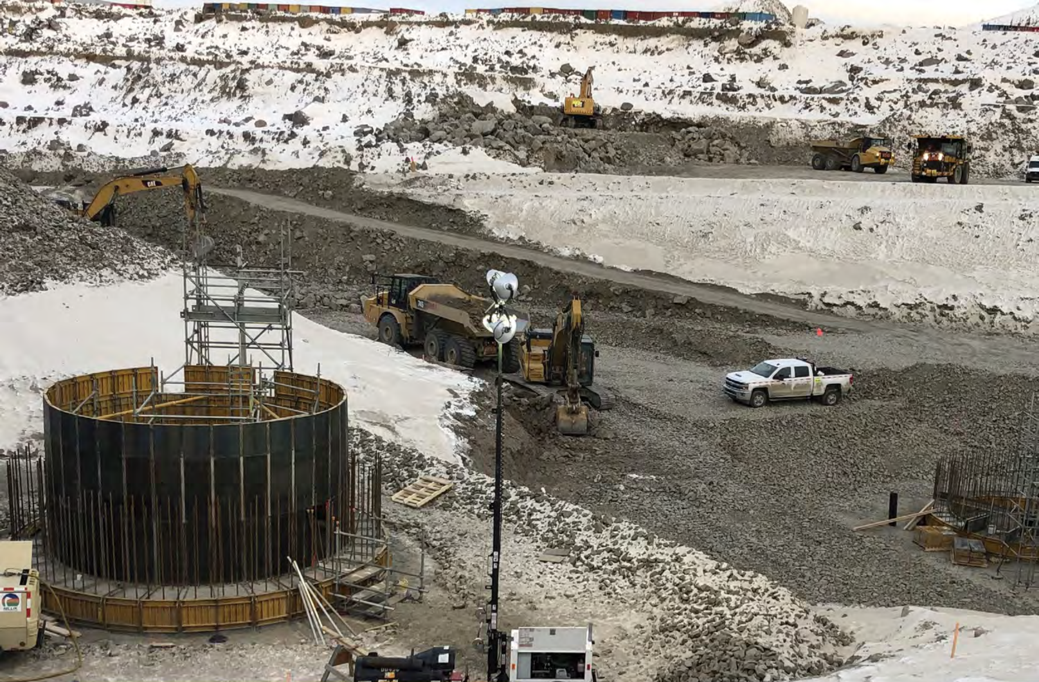
Construction of Raise Bore Collars for the Vale underground mine. (Photo: Timmiak Construction Limited)
