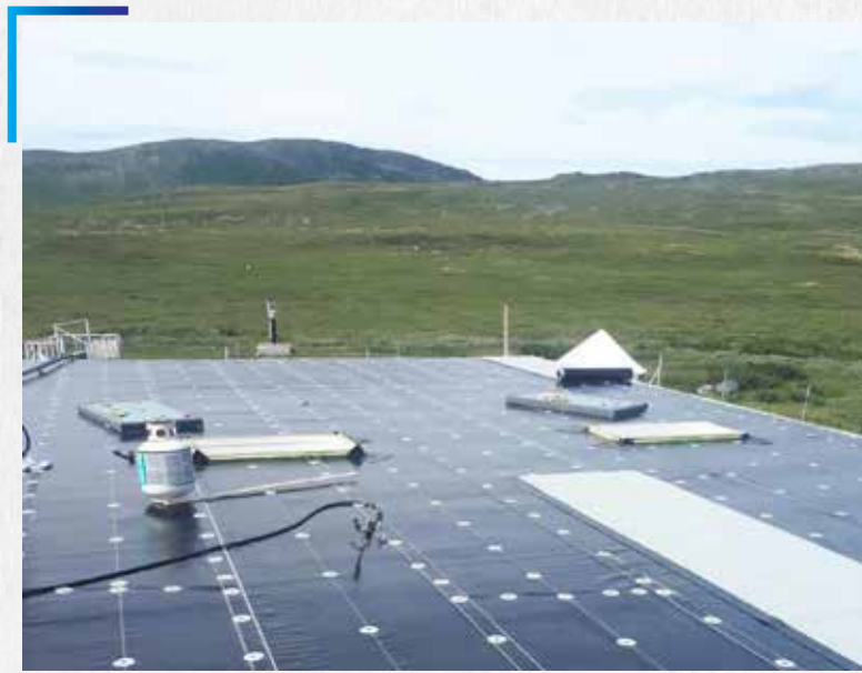
NCI installed a new roof at the Base Camp and Research Station at Torngat Mountains National Park. The company plans to pursue certification in commercial roofing installation. (Tom Lyall photo)
