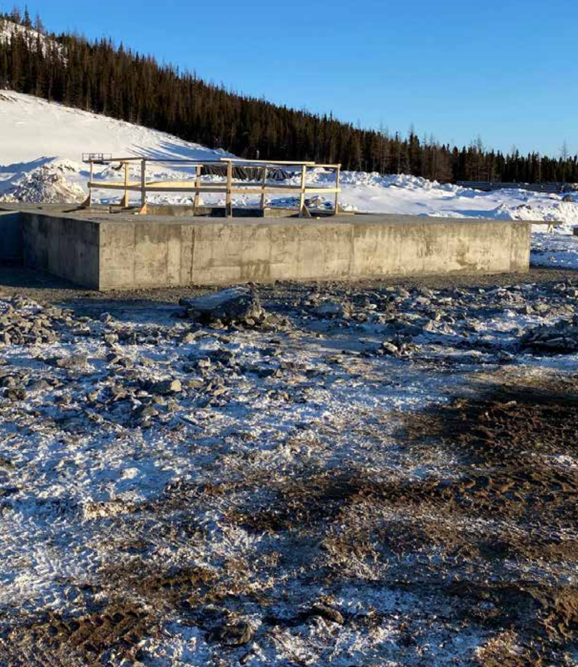
At right, one of five Raise Bore Collars under construction by Timmiak at the Vale site. At left, the surface view of the project. (Timmiak Construction Limited photo)
