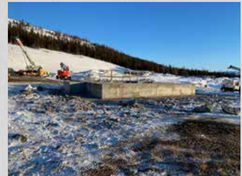
Raised Bore Collar under construction (top) and upon completion (bottom). (Timmiak Construction Limited photos)
