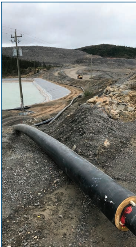
One of the Nillik-Bird Construction projects involves installing a system of water lines and booster pumps for use underground at the Vale underground site. Photo by Nathan Higgins
