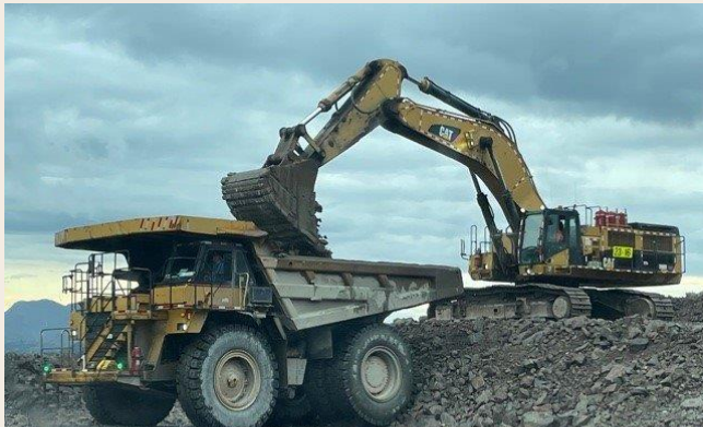
To keep up with the demand for additional rock crushing, Vale asked TSI to provide extra crew to supply rock to the crusher.
