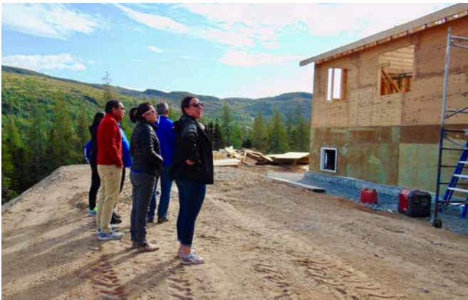
Catharyn, foreground, and Trustees tour a Nunatsiavut Construction Inc. site in Nain.
