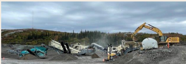
The crushing operation at Vale operates with 11 pieces of equipment and 36 employees.
