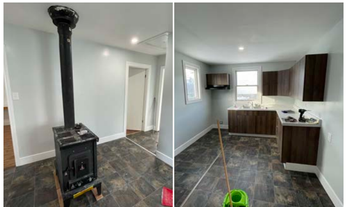
The Home Repair Program includes interior work such as heating, kitchens, and bathrooms, as well as exterior work including roofing and siding. (NCI photos)
