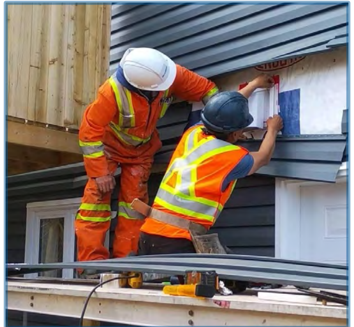
Bobby Williams' crew at work on a siding job in Rigolet as part of the home renovation program.
