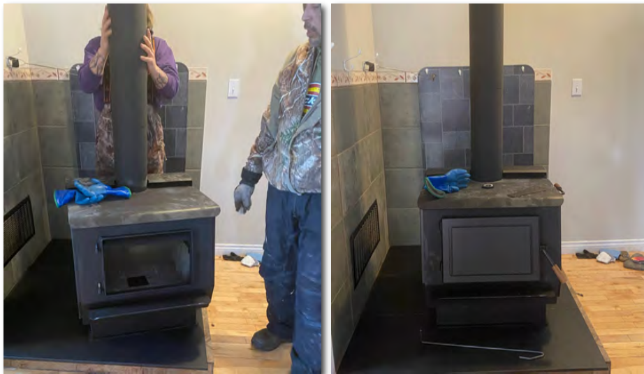
Installers Bobby Williams and Chad Rose put the stove in place, and reattach the chimney. From start to finish, the process takes 45 minutes to an hour. (NCI photos)
