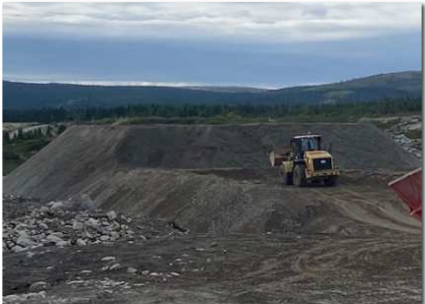
An NCI loader stockpiles aggregate in Labrador City. The company has crushed nearly 100,000 tons of material for Bird Heavy Civil in the past two seasons.
