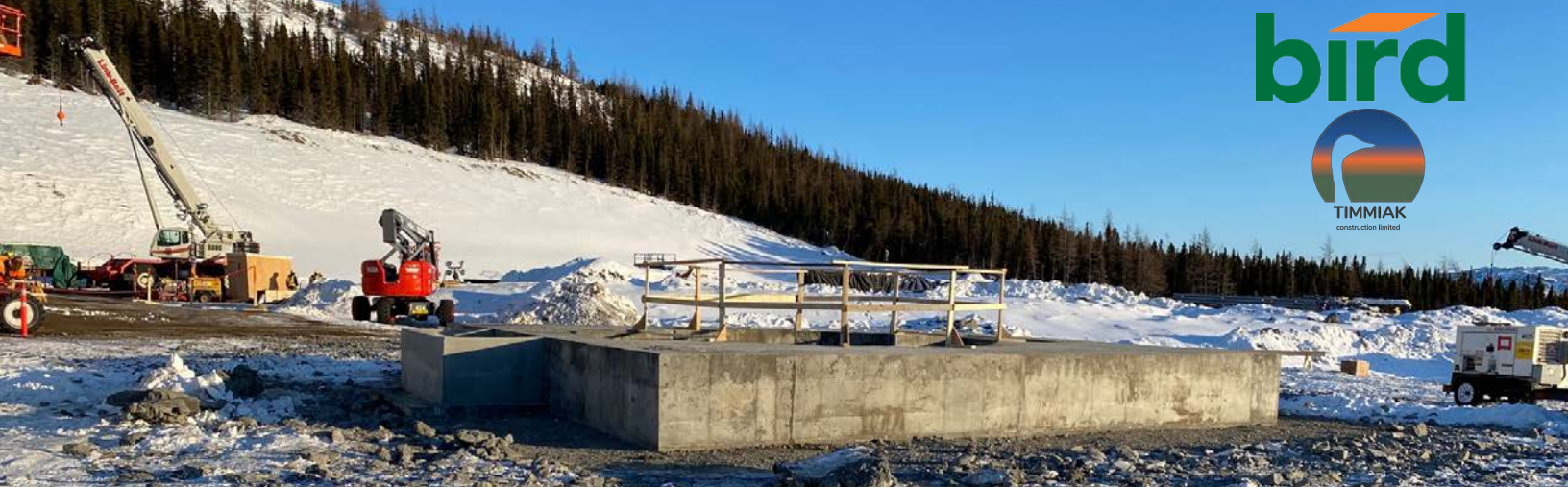
Timmiak constructed five Raise Bore Collars that sit atop mine shafts. Two of the shafts allow fresh air to be pumped into the mine and two will allow stale air to be expelled. A fifth will provide an escape route to the surface for miners. (Photo: Timmiak Construction Ltd.)
